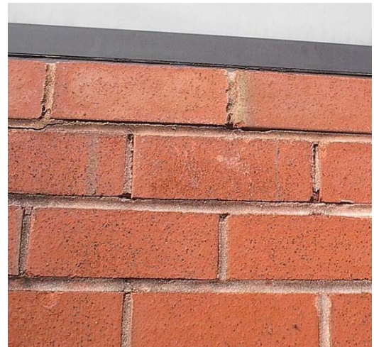
Photo 1 Mortar Joints in Need of Repointing
