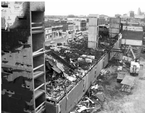
The non-combustible masonry stairwells and concrete first floor are all that remained after the enormous blaze that engulfed the rest of the VCU dormitory on March 26th.
